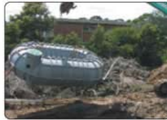
Step 3 Lift tank into hole using lifting lugs on top of tank.
