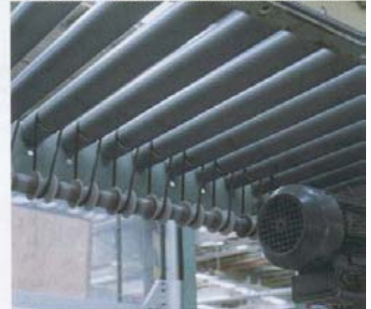
UNDER VIEW OF LINESHAFT CONVEYOR
