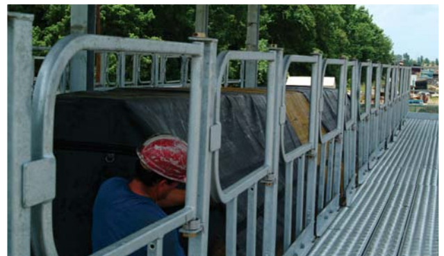
Swing gates help prevent accidental falls
