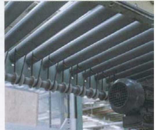
UNDER VIEW OF LINESHAFT CONVEYOR
